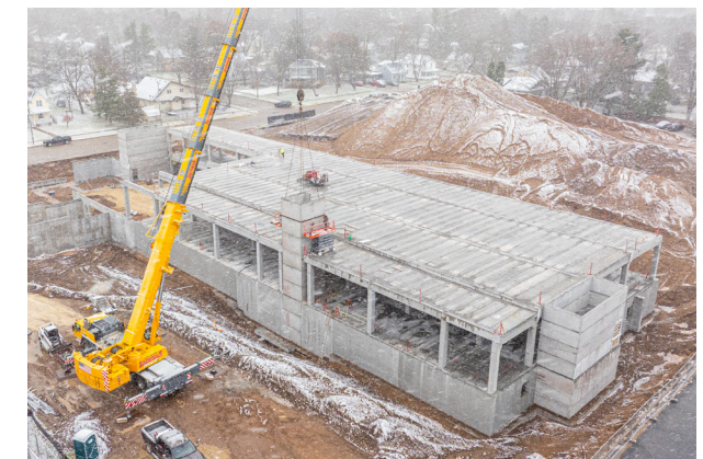
A crane installs precast podium components to form a structural deck, illustrating how off-site manufacturing elements enable efficient placement and accelerated construction progress.
